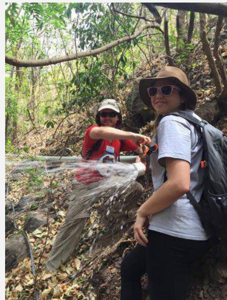
Honduras on a volunteer trip with Global Water Brigades, helping install clean water infrastructure in a small mountain community.
